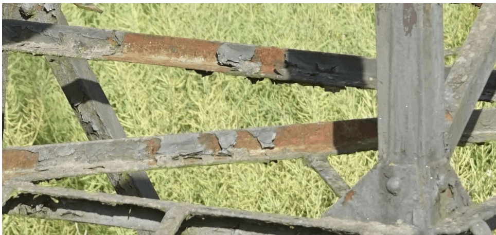
Figure 2.1: Corrosion of on an electrical tower (image provided by Axians).
